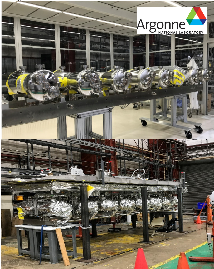
HWR cryomodule cold mass assembly
