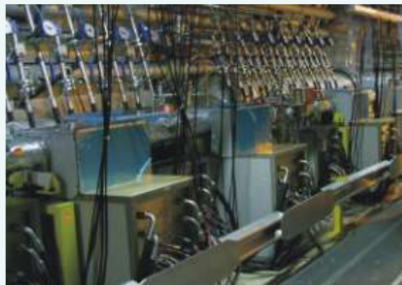
Electrostatic Kickers and Wideband Power Amplifiers in the LHC tunnel
