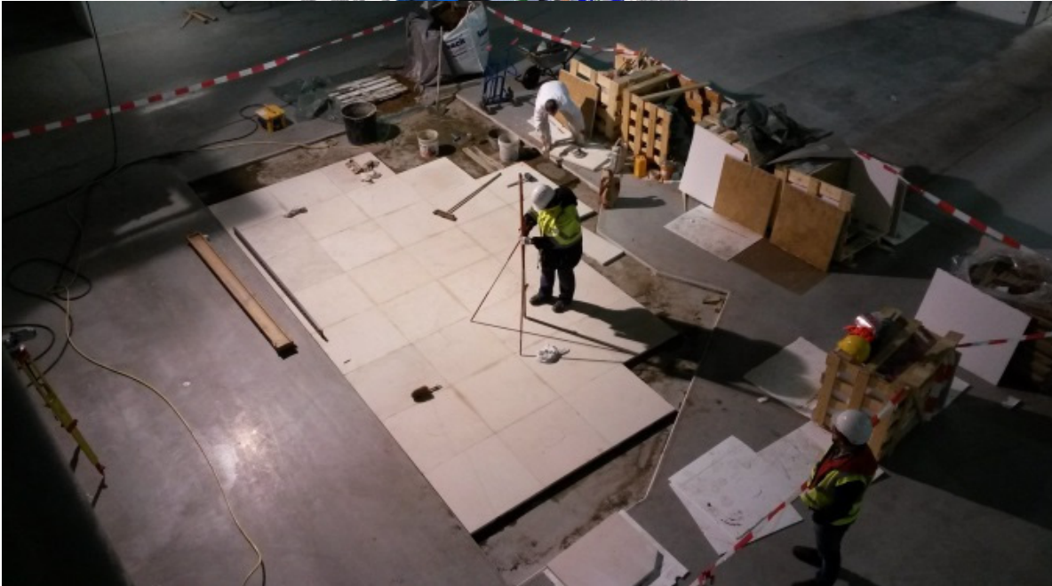
Integration of high-precision floor into normal concrete (civil construction vs. fine polished floor)
