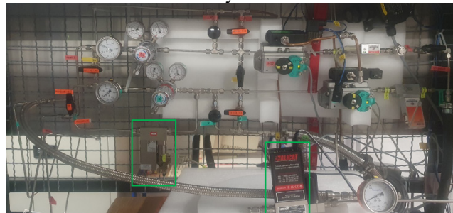
Figure 5: Photo of the gas control station with the two electronic pressure controllers that were successfully tested during the beam time.
