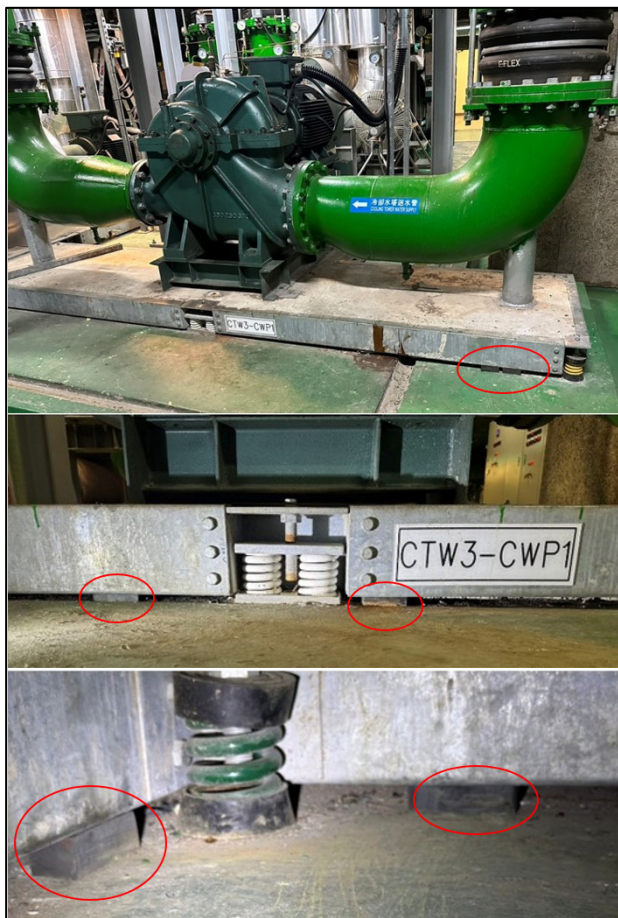
Figure 3: Strengthened structure of the CWP-1 system, with hard rubber installed between the concrete basement and the ground.
