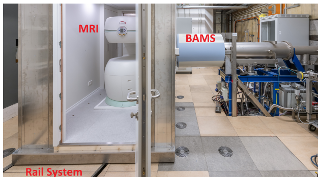
Figure 3: MRI installation on its rail system.
