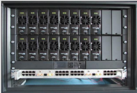
50VDC Eaton Power supply
