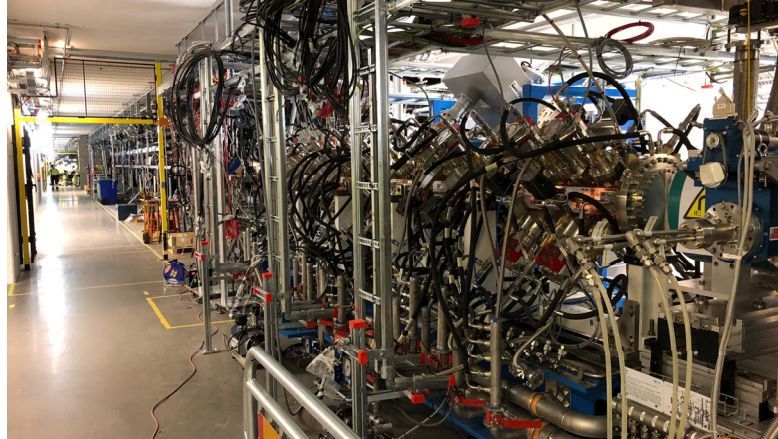
Parts of Normal Conducting Linac Under commissioning
