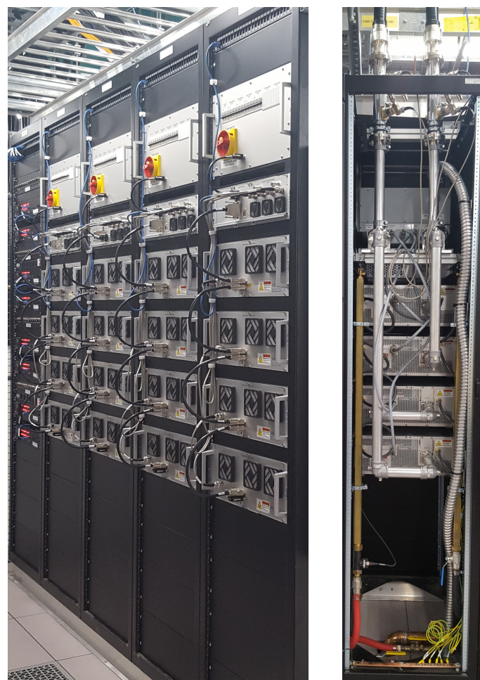
80.5 MHz RF Amplifiers in LS1
