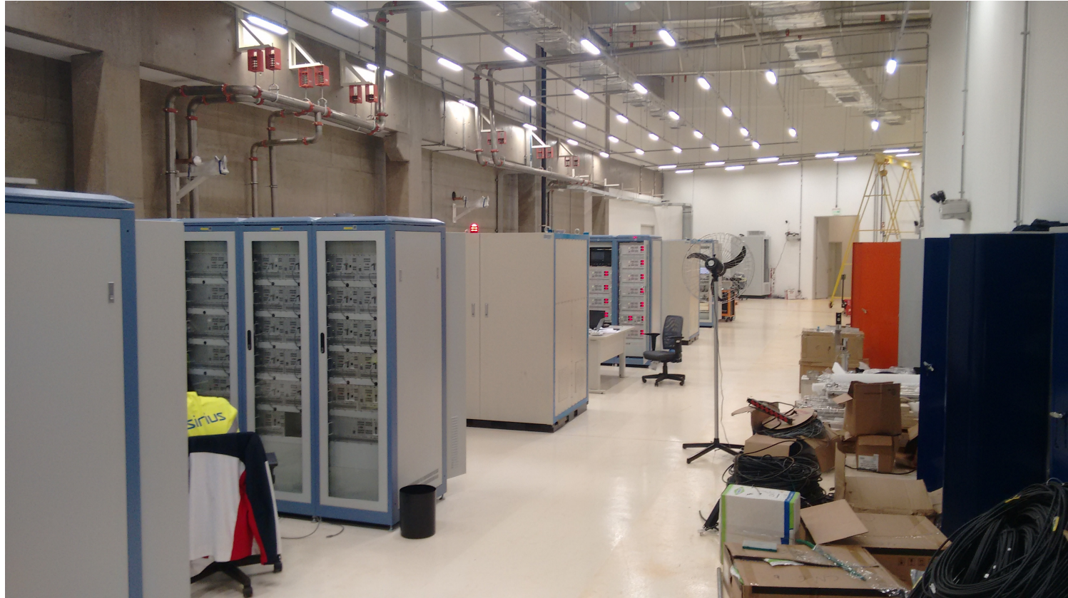
LINAC klystron room during installation
