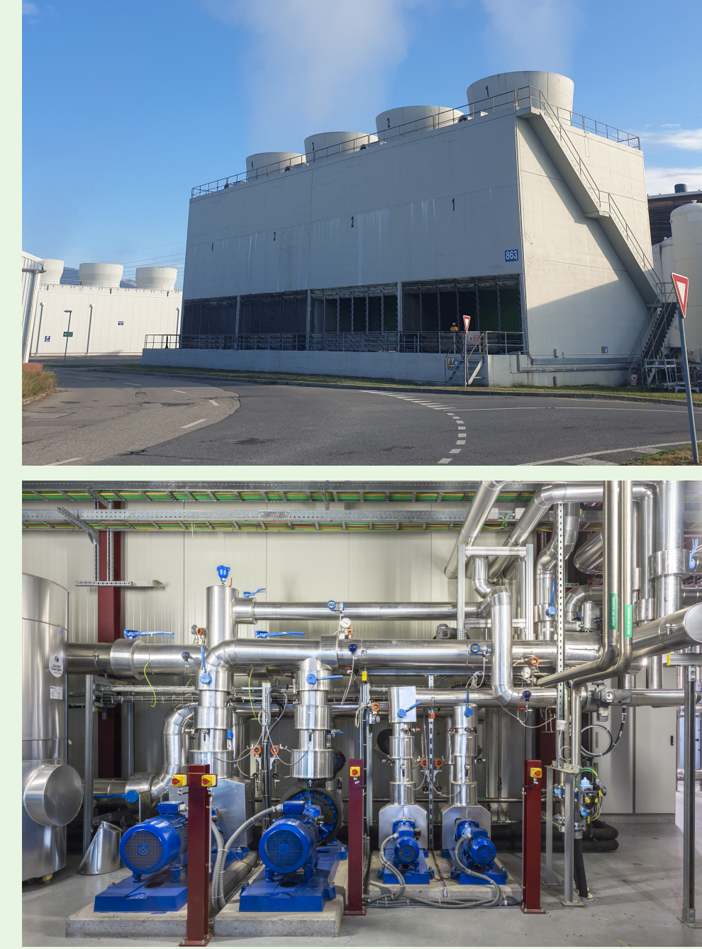
Figure 1: Cooling and ventilation plants at CERN
