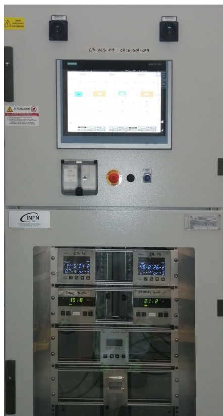
Figure 5: VCS Rack installed in ALPI.
