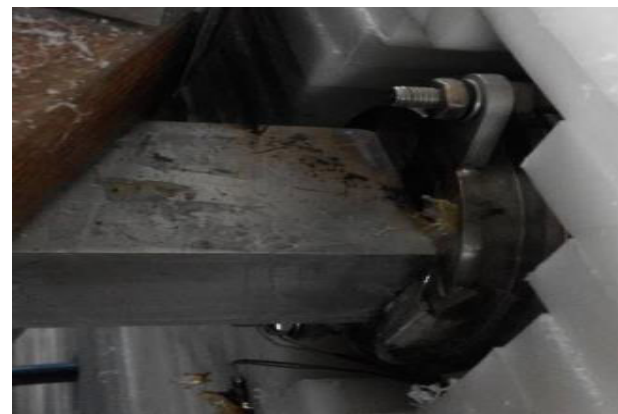
vacuum pipe of bending magnet 2.7mA@2.5MeV, CW, 1min
