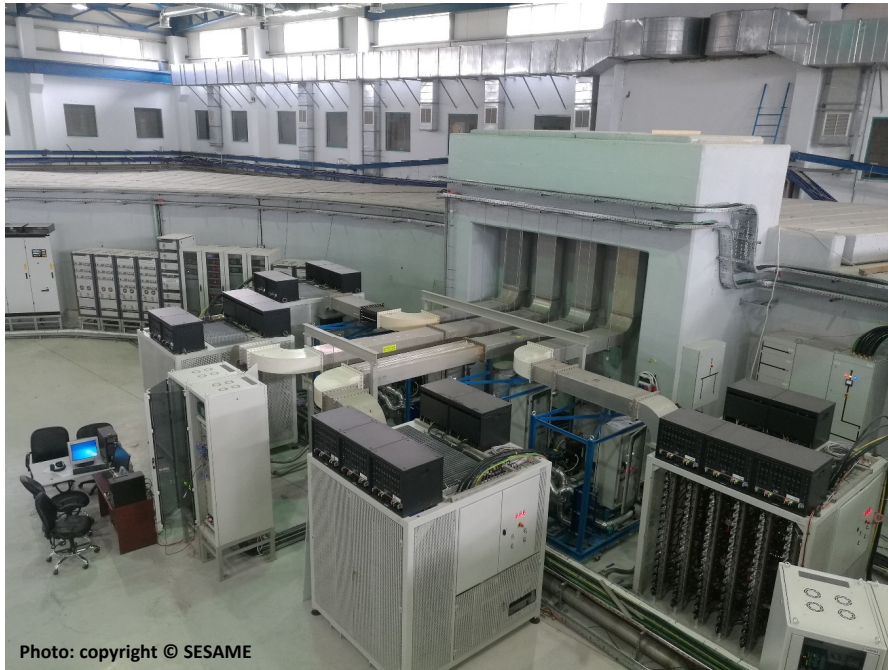
RF Plant (4*80KW SSA)
