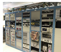
Equipment racks in the BLIP control room
