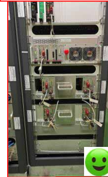
New power converters for steerers and A/q separator
