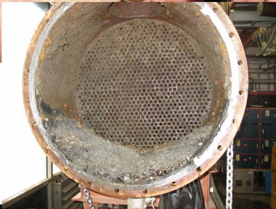
Main Injector heat exchanger pipe clogged by mussels
