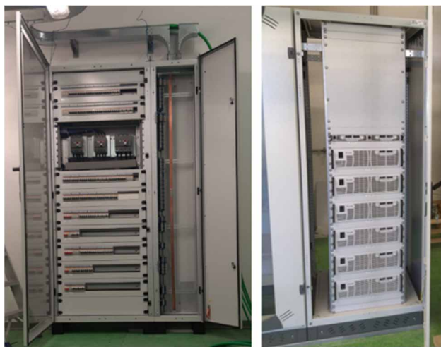
Figure 2: On right side, the picture shows the new main local electrical board dedicated to supply the cyclotron's components. On the right side the new cabinet with the power supplies of LARMAED beamlines magnet.
