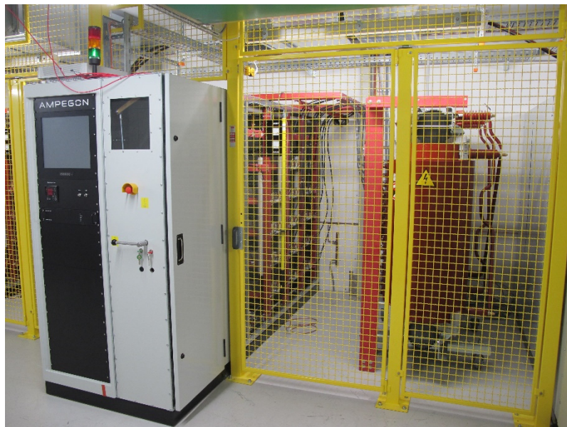
APS Ampegon 15kV, 40A
