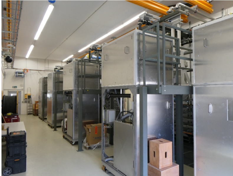
Power amplifiers installed on ground floor in WHFA
