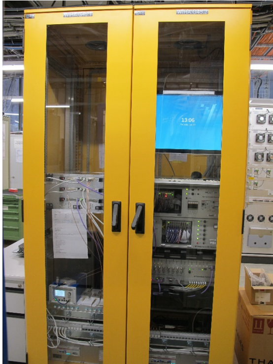
Installation for new LLRF system
