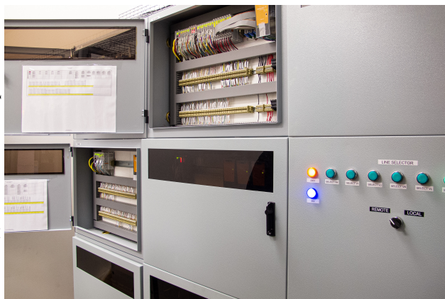
Figure 3: Unistrut EtherCAT cabinets designed at iThemba LABS.
