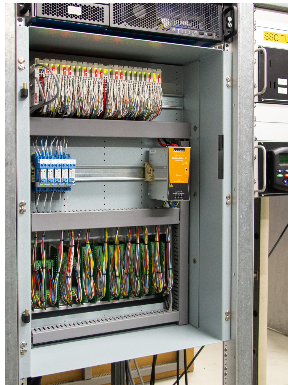
Figure 4: Custom 19-inch rack mountable EtherCAT cabinets designed at iThemba LABS.
