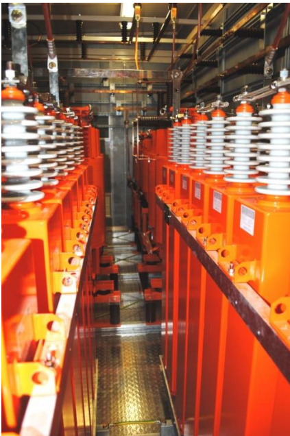
New power grid filter delivered mid of 2013
