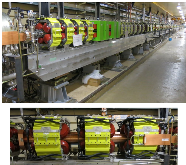
Figure 6: Densely placed quadrupole magnets for transportation of large emittance positrons. They are overlapping with the accelerating structures.
