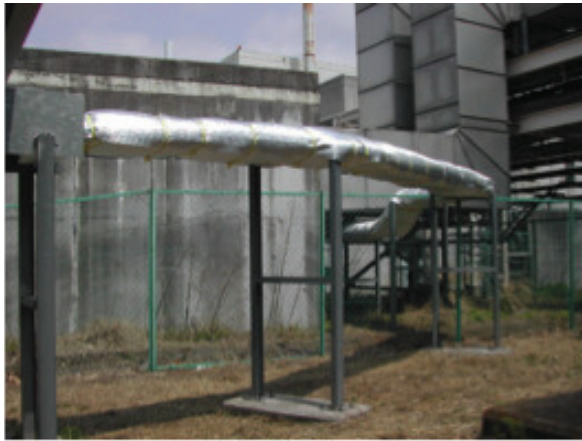
Figure 8: A thermal insulator sheet for BPM cables installed near the local control building (LC4).
